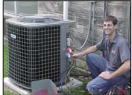
Joe Cantelli of Sun Ray demonstrates ease of access to electrical panel and service ports for checking pressures and sub cooling on the Comfortmaker N4A3 5 ton unit.
