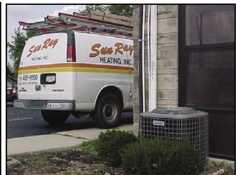
2½ ton units for each classroom are positioned close to the air handler for short refrigerant lines. School staff was impressed with the low sound levels of the outdoor Comfortmaker units.
