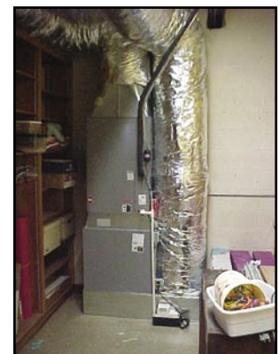
Spiral Duct provides three supply registers and single return for each classroom served by a 2½ ton system.
