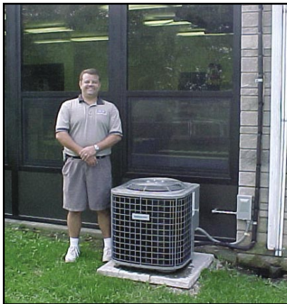
Bob Krause of Sun Ray takes pride in providing a quality installation and system upgrade for Immanuel Lutheran School.
