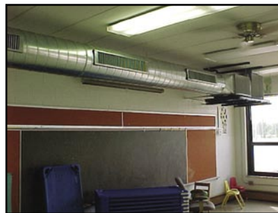
Shop fabricated return box and coil transition make good use of limited space available.
